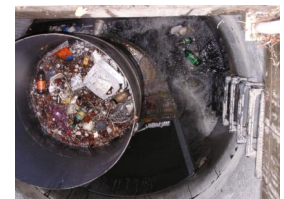
Inside a storm drain filter
