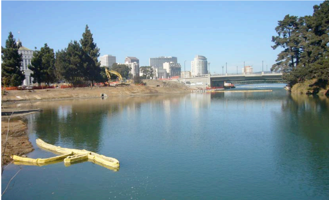
Former fill was removed from the area to the left of the channel. The new marsh will be exposed at low tide. (photo courtesy of Joel Peter)
