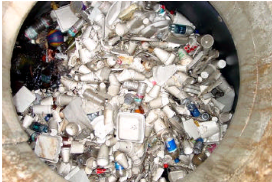
Looking down into the storm drain filter at Valley and 22 nd Streets.
