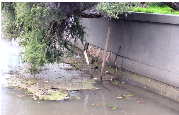
Water about 3 feet higher dislodged the barrier.
